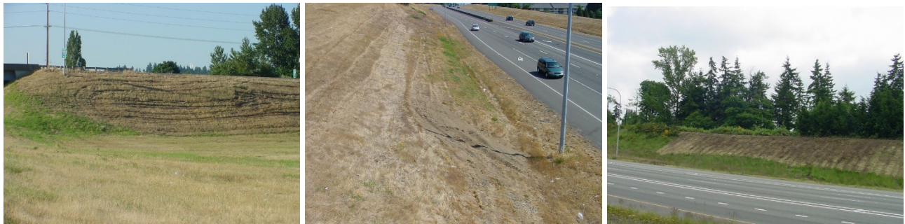
Figure 8. Mower damage on slopes (Courtesy of WSDOT).
